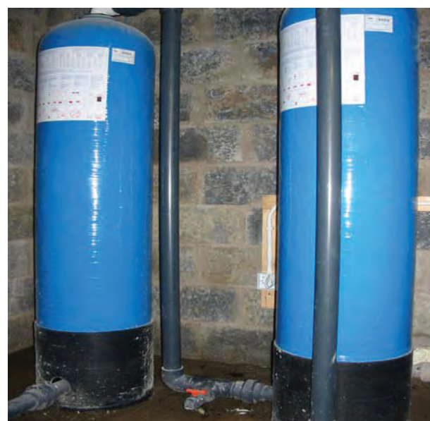
Figure 1.5 Specialist Arsenic Removal Filters
