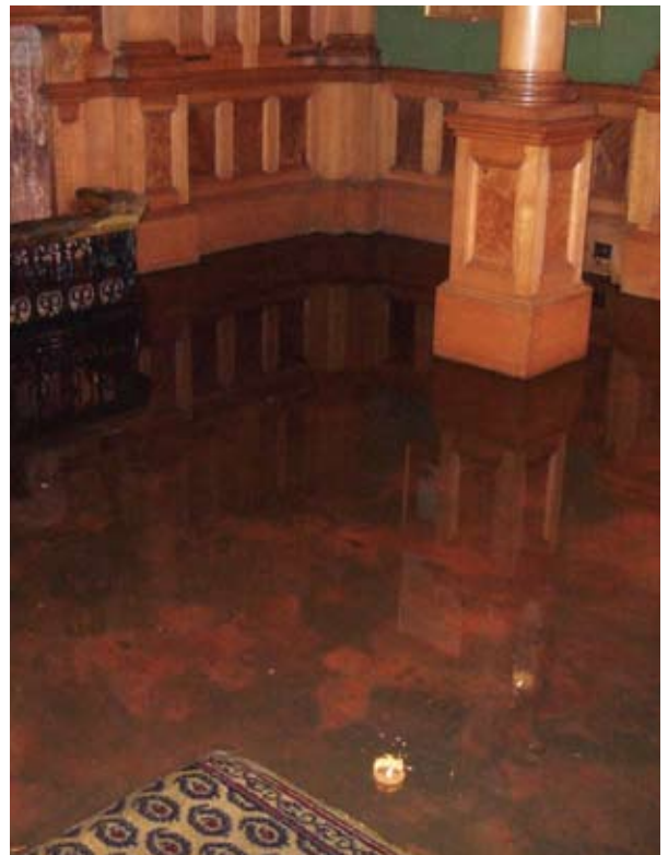
Craggside, Northumberland, Billiard Room under water
