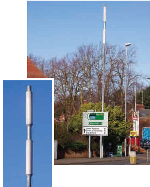
An example of a slim-line monopole. A simple well-proportioned installation.
