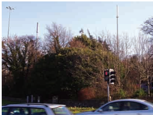
Masts located within a group of trees at a major traffic junction
