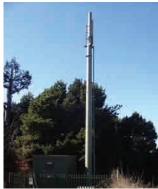
Equipment cabinet adjacent to a monopole mast.
