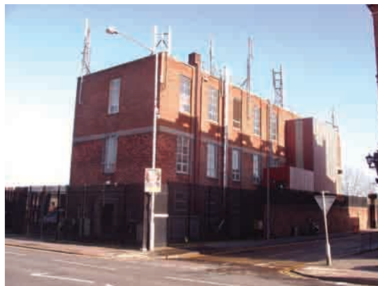
An example of a rooftop cluttered with antenna.
