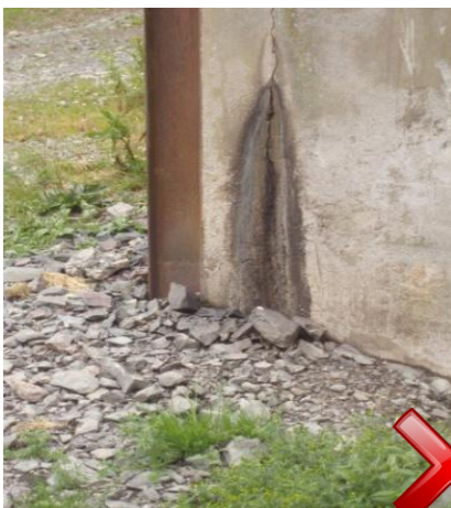
Photo 6 - Leaking silage clamp
