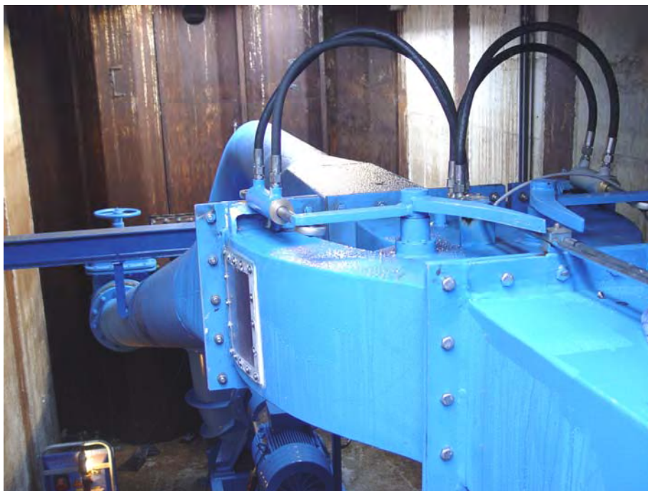
Figure F5.15. Part of the structure of the “Fishway for pumping stations”. The pumped flow comes along the pipe in the centre of the photograph. The flow containing the fish comes up pipes on either side; one can be seen on the left. Photograph courtesy of Fish Flow Innovations.
