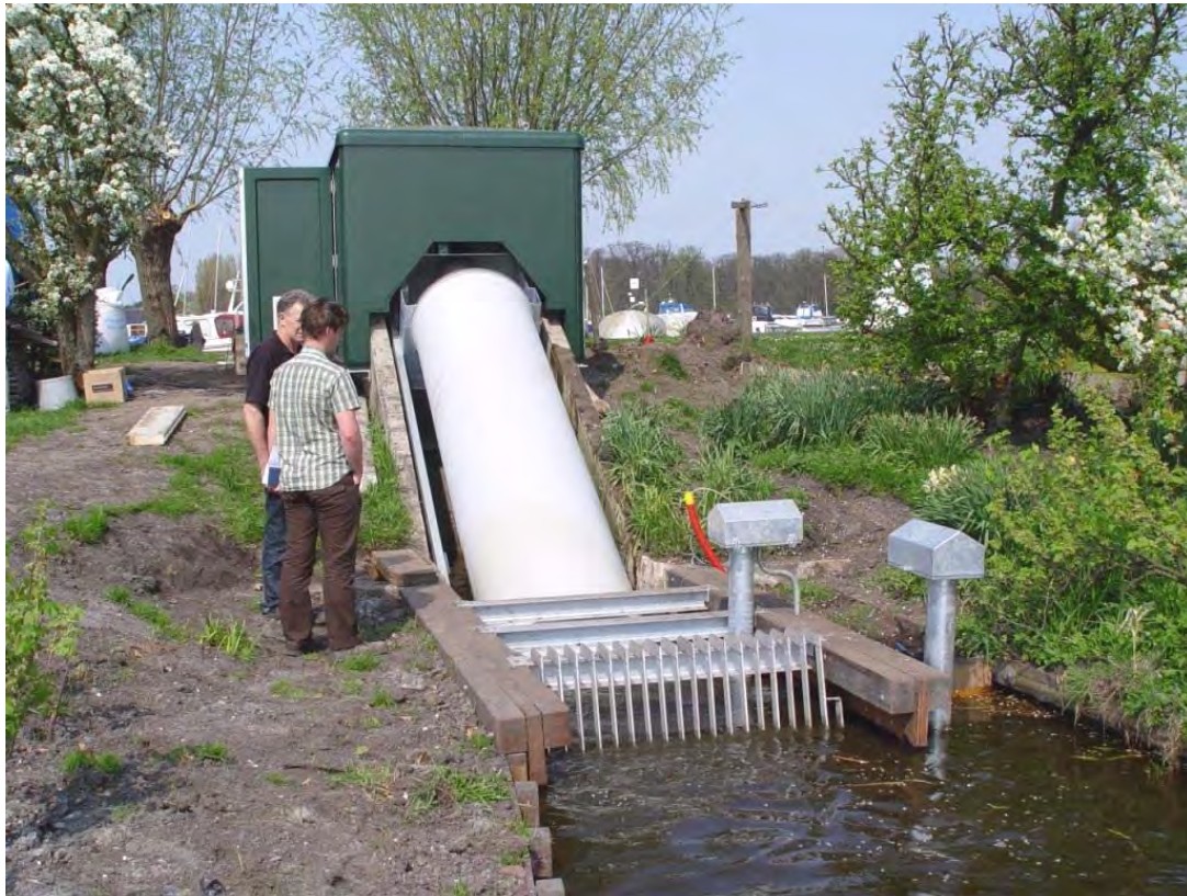
Figure F5.10. Fish Flow Innovations Archimedes screw pump at a pumping station at Zwanburgerpolder, Netherlands. Photograph courtesy of Fish Flow Innovations.
