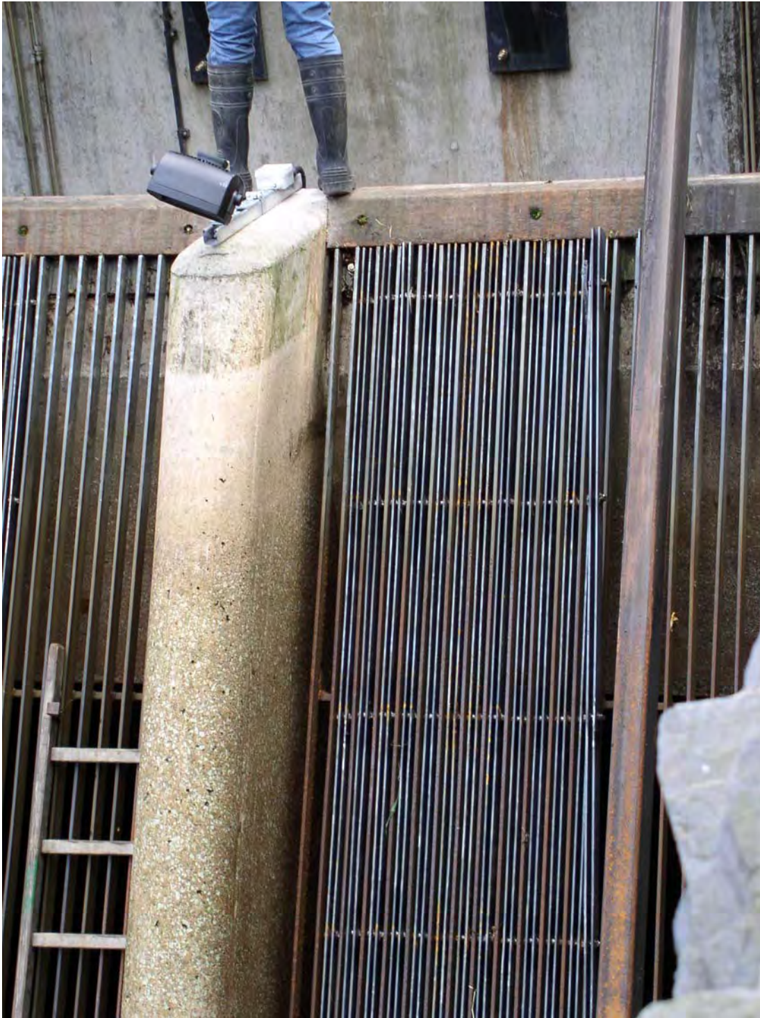
Figure 4.3: Vertical bar racks being overlaid with additional bars to reduce the effective bar spacing. The photograph was taken at the Backbarrow hydropower scheme in Cumbria during the process of adding bars and is incomplete as shown. The overlay screens only remain in place during the autumn eel migration season.
