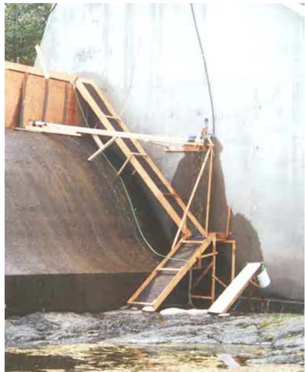
Figure 6.6. Pumped-supply pass at Fort Halifax Dam. A “portable passage” ramp (see Section 6.6.4) is being deployed alongside. Photograph G Wippelhauser.
