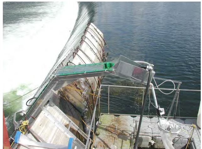
Figure 6.8. View of Chambly Dam eel pass from above. Note covers over the channel containing the substrate, and the electronic counting device on the pipe carrying the eels from the top of the pass to the keep net. Photo D. Desrochers.
