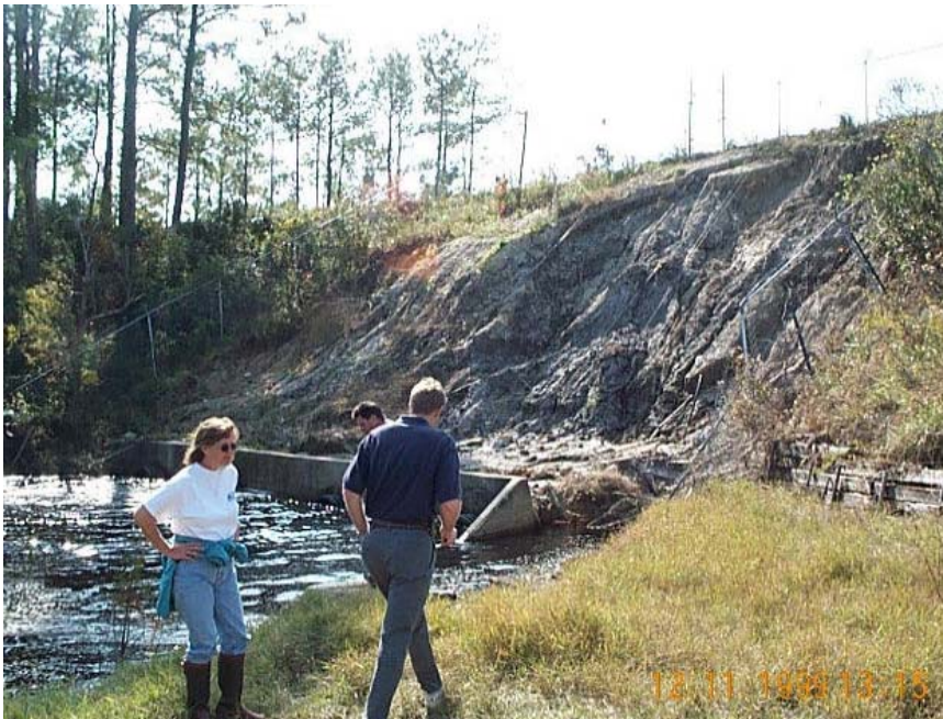
Figure 3.53 Instability of downstream shoulder of dam (North Carolina Department of Environment and Natural Resources, 2009).
