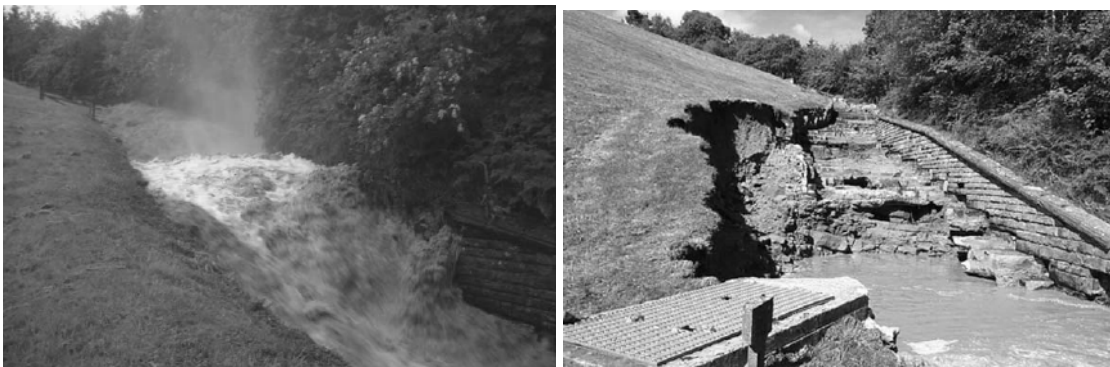
Figure 3.54 Flood event of June 2005 that resulted spillway damage at Boltby reservoir (Walker, 2008).
