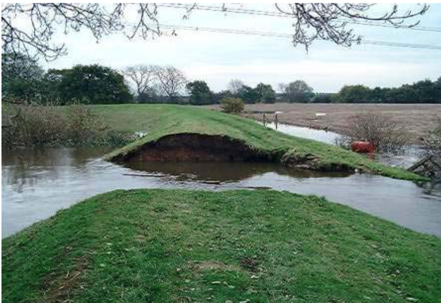
Figure 3.48 Dam breach (Morris, 2009b).
