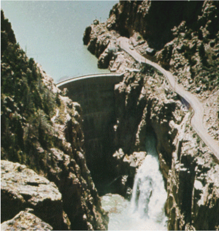
Figure 3.49 Foundation failure of concrete dam (Durham University).
