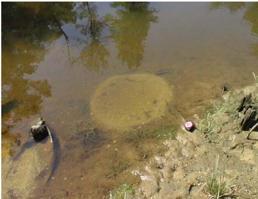
Figure 3.56 Muddy discharge downstream of dam as a result of increased seepage and internal erosion (North Carolina Department of Environment and Natural Resources, 2009).
