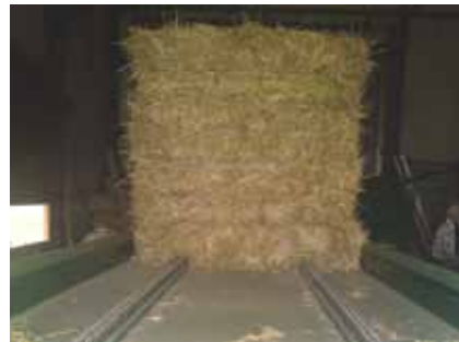
Whole bale boiler being fed into shredder prior to entering the combustion zone
