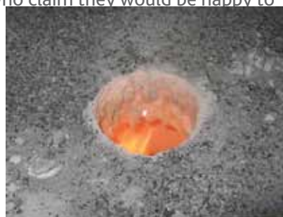
Clinker building up around the heat exchangers. This is often solved by adding ground limestone.
