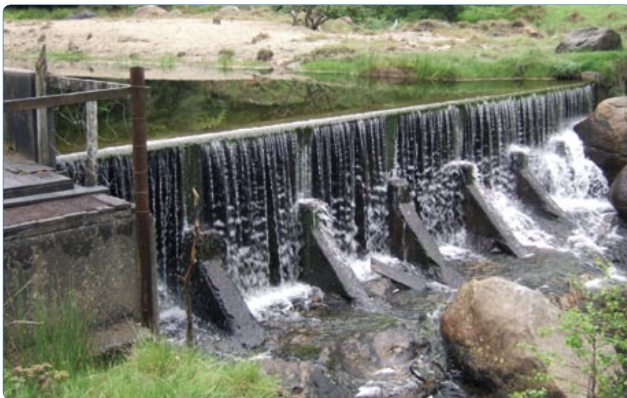
Obstruction to upstream fish passage.
