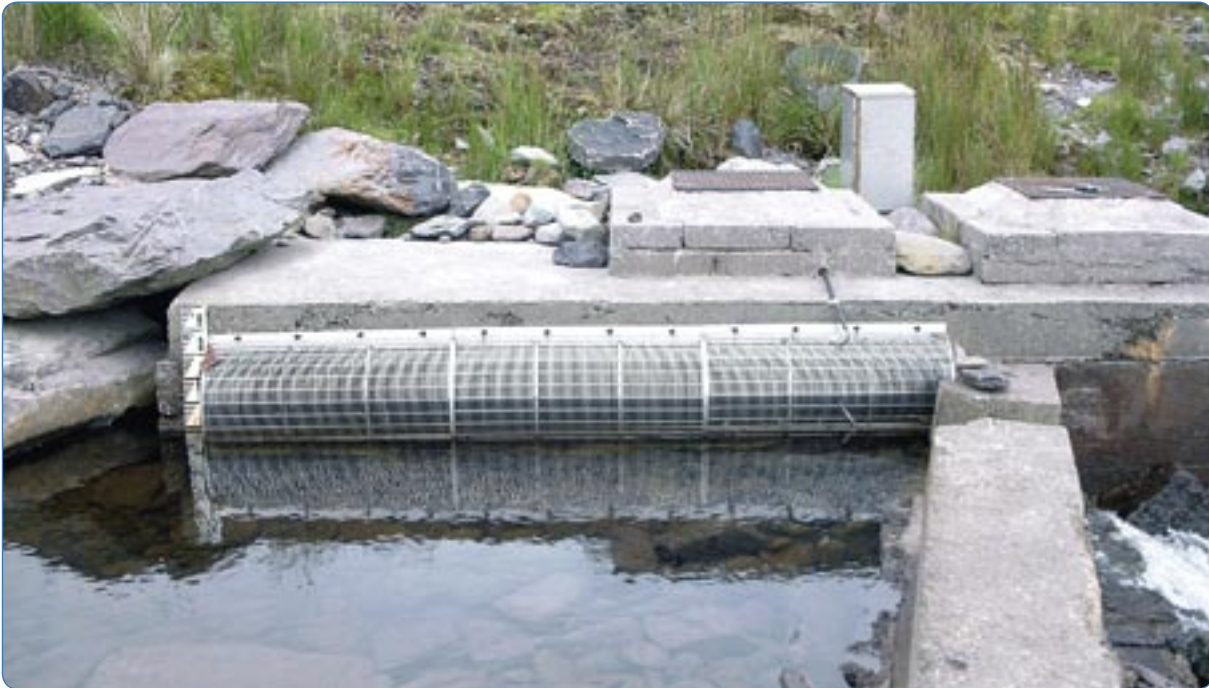
Intake screen arrangement at a high-head site.
